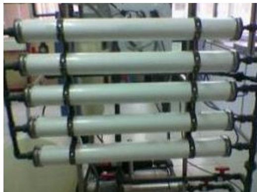
Pilot Scale RO Plant
